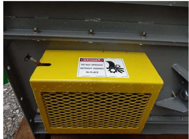
Secured fixed guard on rotating shaft end
